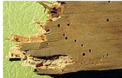
Powder post beetle damage to wood
